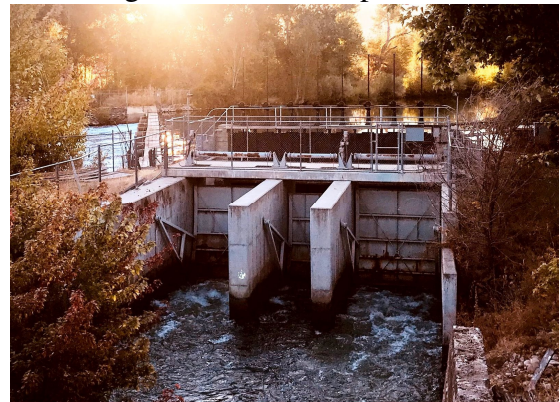
NMID’s Boise River diversion headgates.
